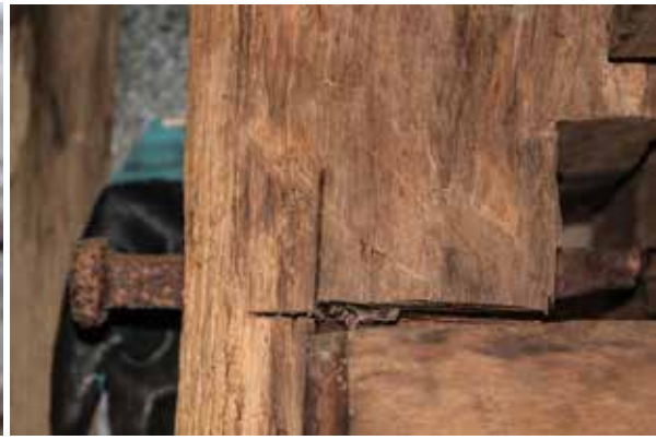
Figure 82 View of bolt, broken at screw thread
