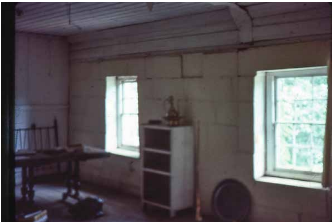
Figure 66 – First floor, with north-facing windows on right and internal wall on left
