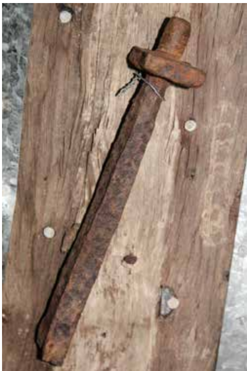
Figure 79 Bolt with broken head
