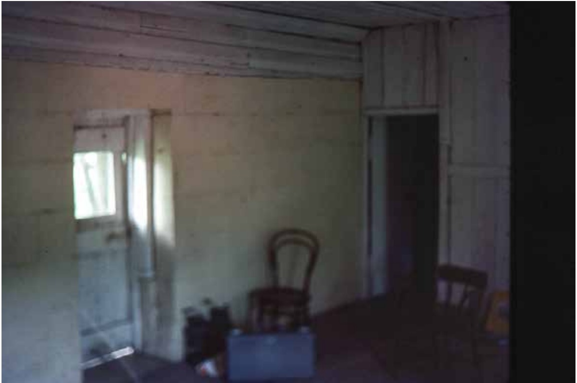
Figure 65 – First floor, with door to verandah on left and internal wall to eastern room on right
